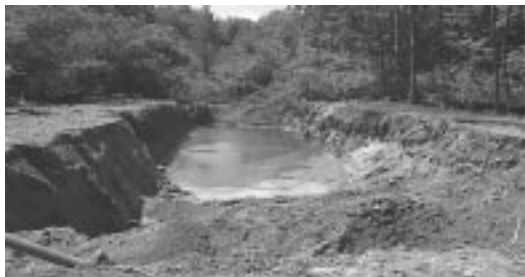
Based on test results and RAB recommendations, Westover's contractors excavated potentially contaminated areas behind the former Jet Test Stand due to concerns about contamination.*
